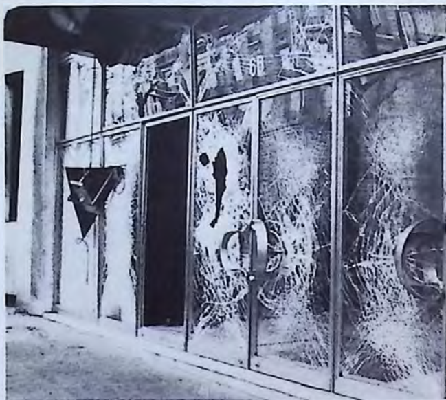
Damage to the doors of the building, while extensive, was somewhat reduced by protective materials added after the previous attack.
